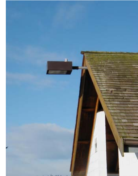
Appropriate Shoe Box Lighting (Sodium Light) on the side of a building:
