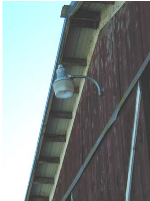
Non-Compliant Mercury Vapor Light:
