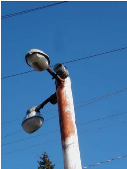
Non-Compliant Parking Light:
